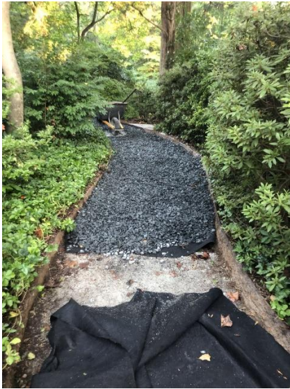
Fabric being laid out over the existing base and covered with gravel
