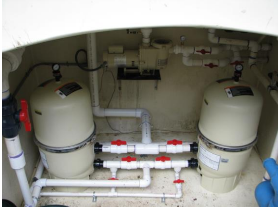
The underground vault with new filtration tanks
